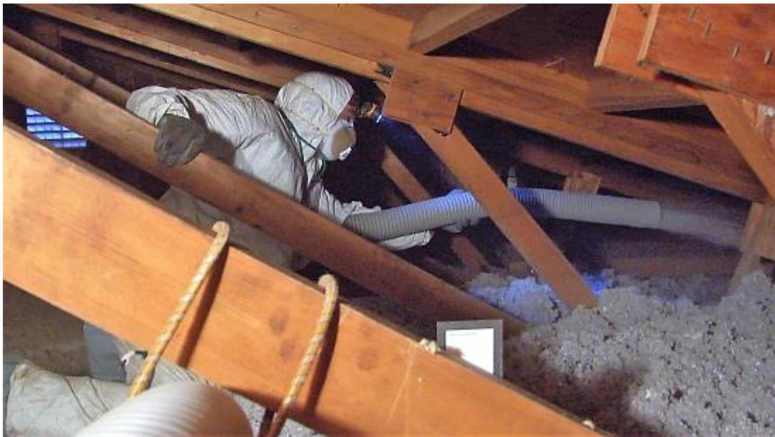
Adding attic insulation to reduce heat loss is one of the primary activities of the Weatherization program.
